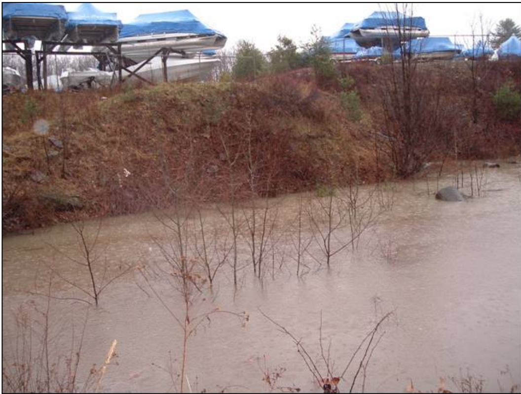
Poorly-functioning Detention Basin Adjacent To Bakker Marine Before BMPs Installed
