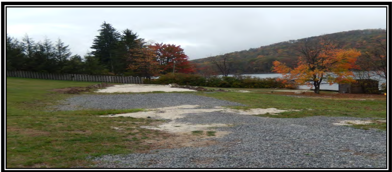
Installation of sand volleyball court, no containment of disturbed soils, directly adjacent to lake
