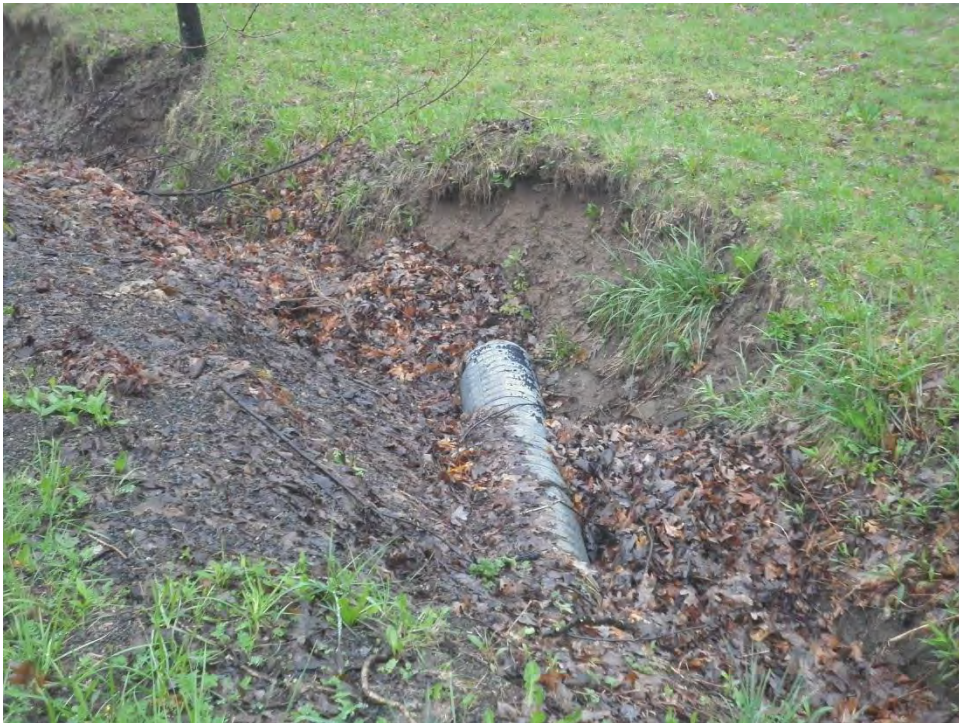
Photo #421 Eroded outfall
