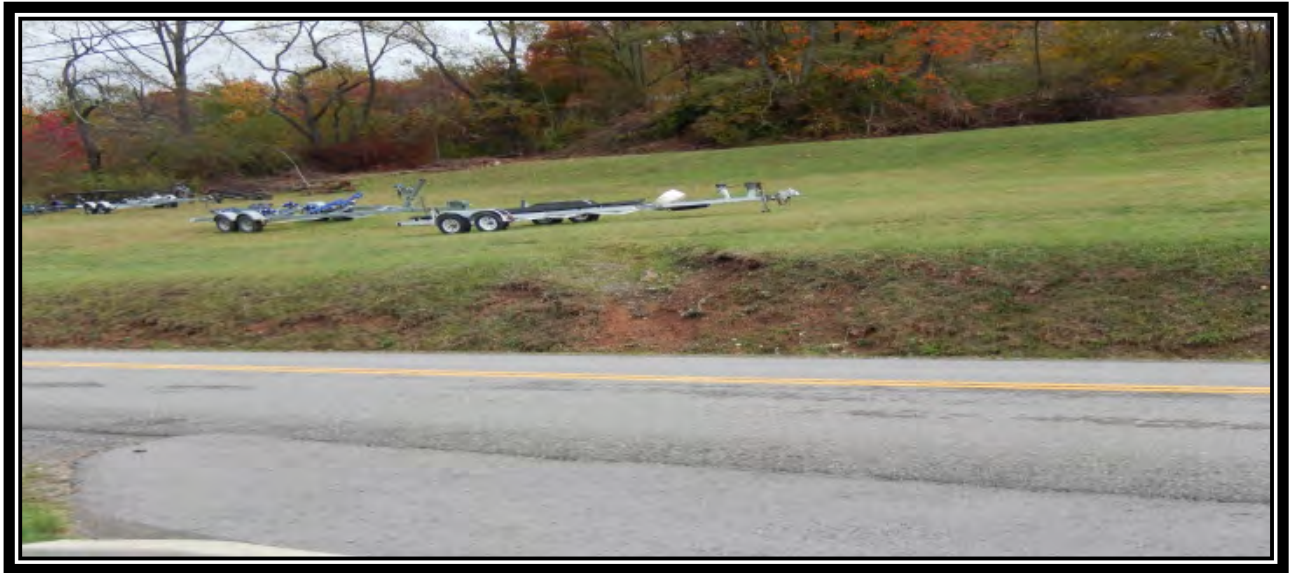
Overflow parking area, slope failure causing erosion
