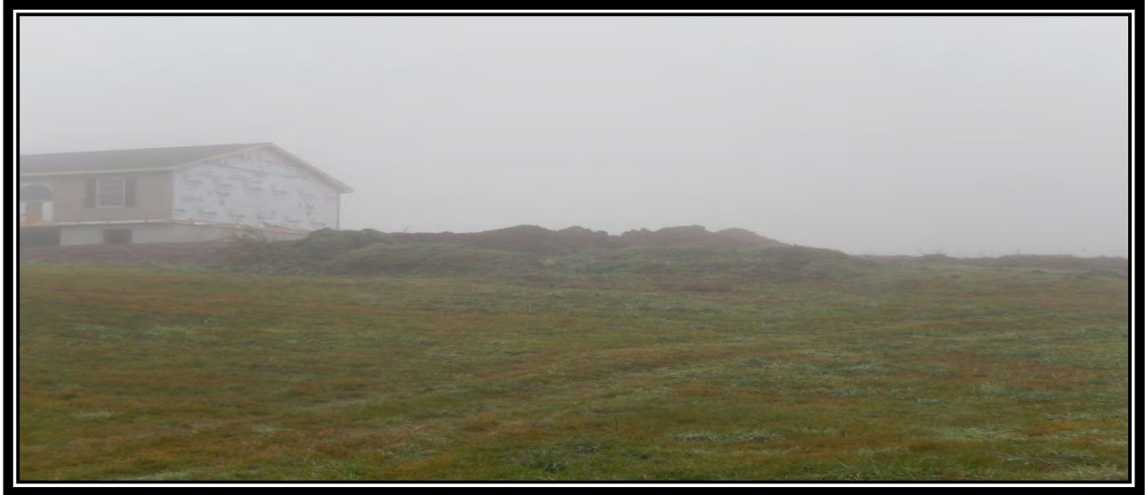
Home Improvement with soil disturbance and no silt fence
