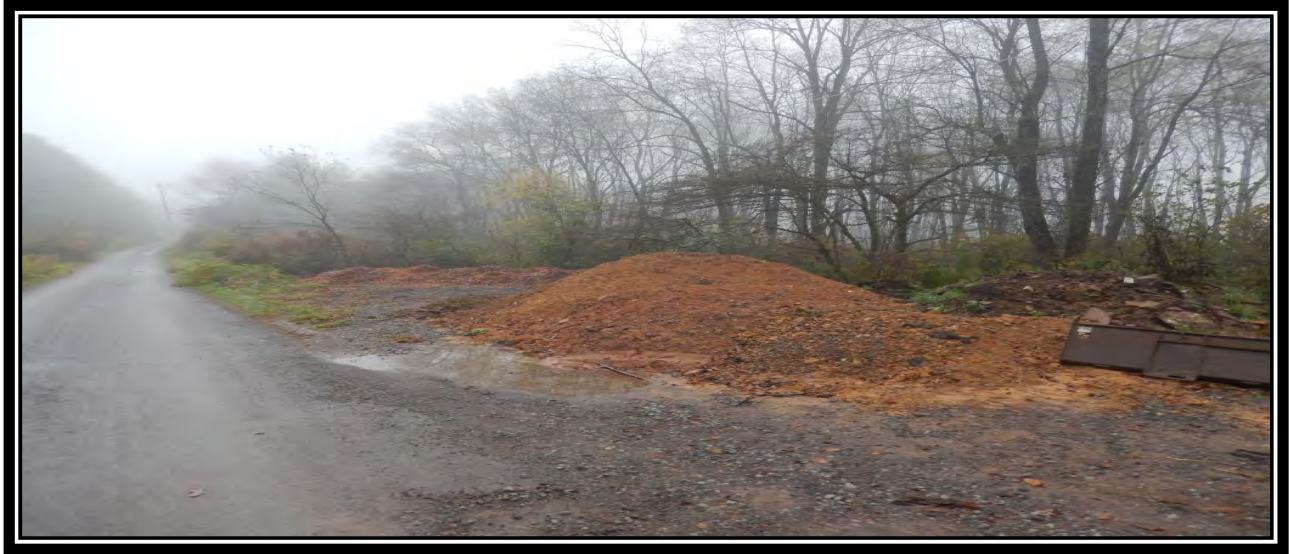
Soil pile from construction, directly adjacent to stream
