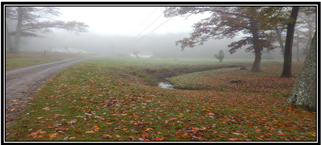
Left bank erosion in tributary stream
