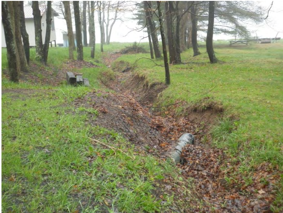
Photo #424 Outfall erosion
